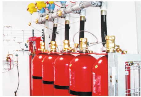
Clean Agent Fire Suppression System
