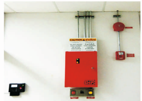
Fire Detection System
