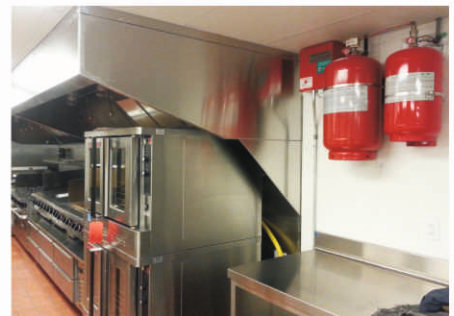
Kitchen Fire Suppression System
